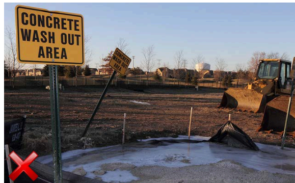
Poor job of containing washout inside of the designed area. Washout material should be removed when capacity becomes an issue.
