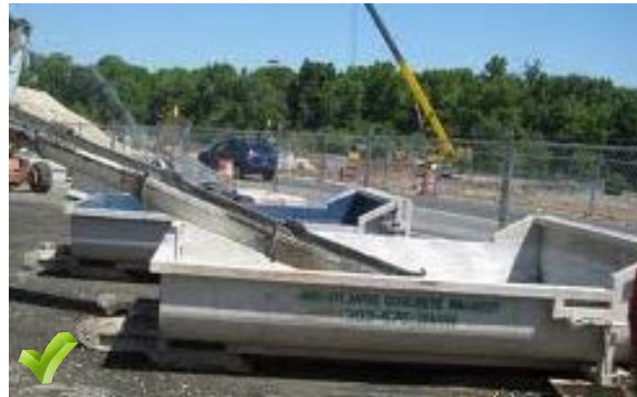
Self-contained sturdy containment systems that are delivered to a site and located at strategic locations for concrete washout.
