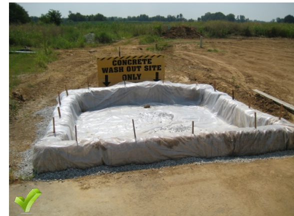
This above grade washout system has the correct polyethylene lining which is wrapped around the straw bales. The washout is underlain with DGA to provide a solid base for the washout and to prevent punctures in the plastic liner. Straw bales are securely anchored to the ground, and a large sign identifies the washout.
