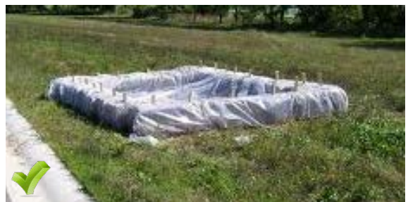
Good example of above grade system with straw bales and a polyethylene lining. A "Concrete Washout" sign should be installed at this location.
