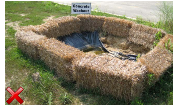
The polyethylene lining should wrap over the straw bales and be properly secured along the top. The lining used at this washout area is not thick enough.
