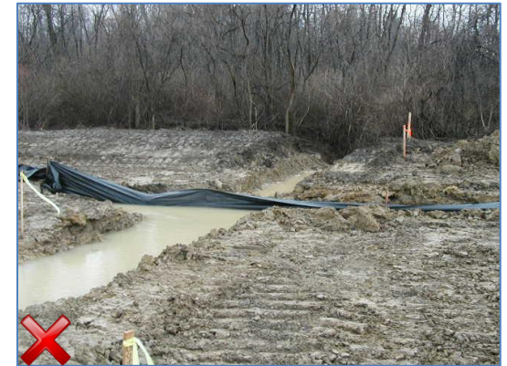
Example of poor sediment trap installation. Silt fencing should never be used as an outlet structure for a sediment trap.
