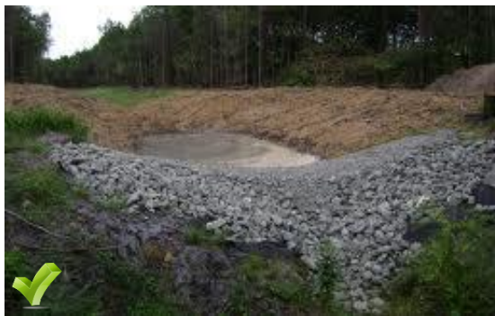
Good example of a sediment trap. Rock overflow notch is properly installed and bare soil has been covered with seed and mulch.
